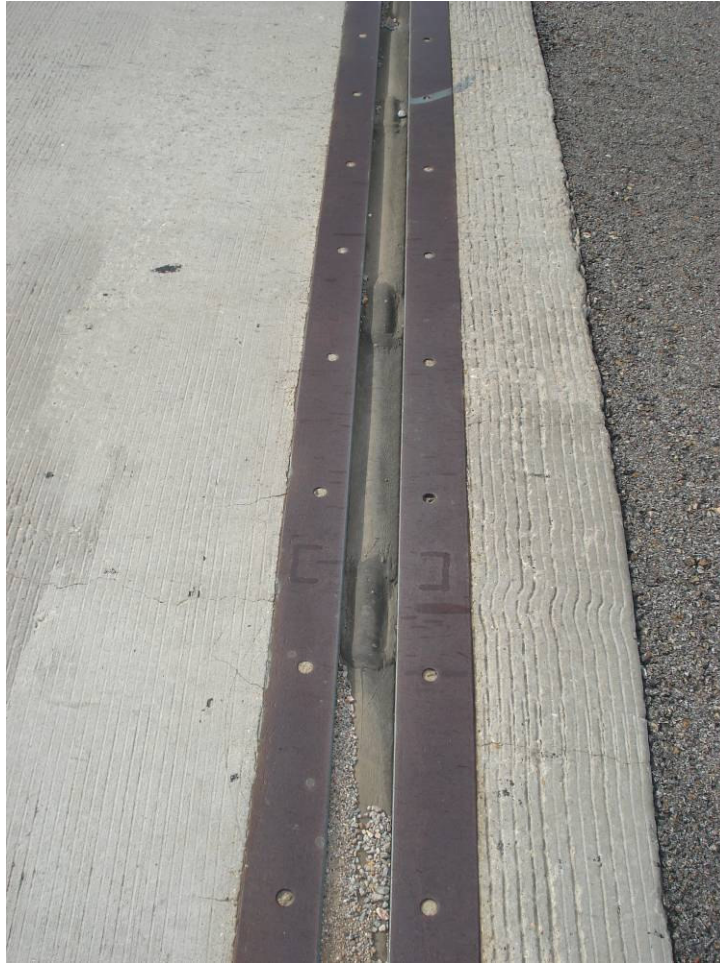
Figure 20: Highway 63 Bridge with Interval Patching
