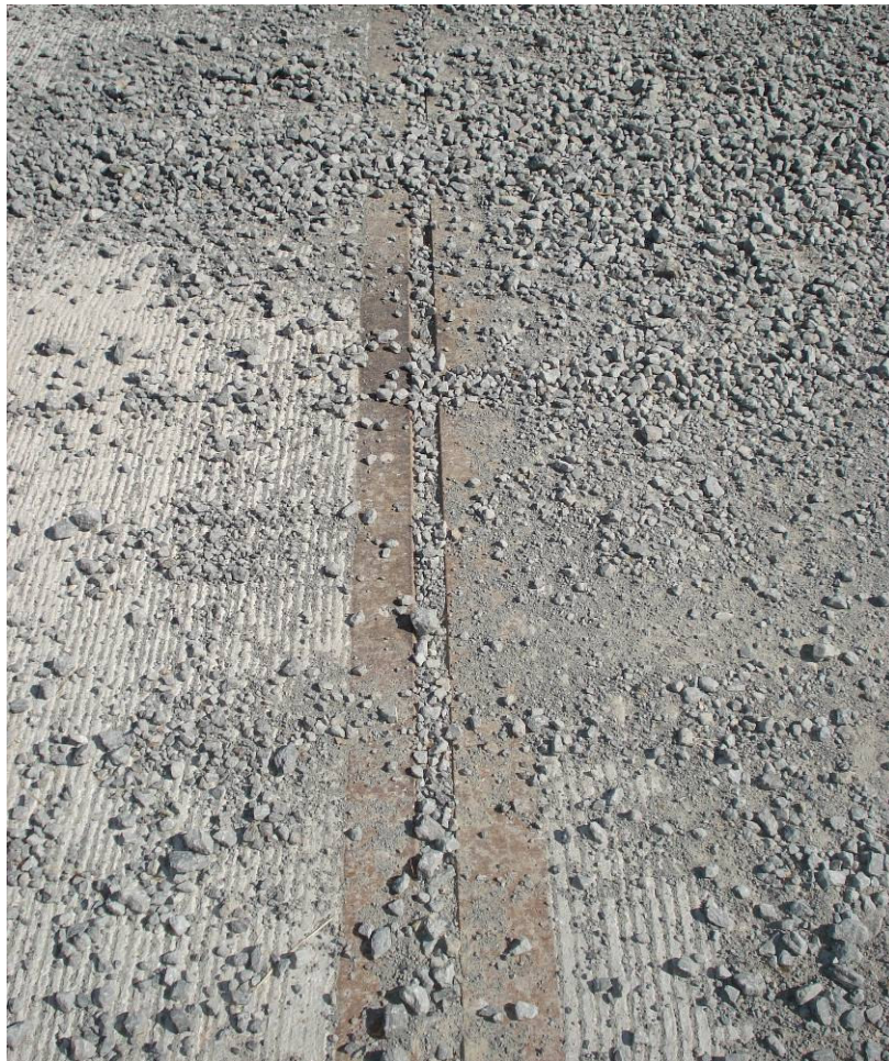
Figure 19: Debris in Joint at Cadron Creek Bridge
