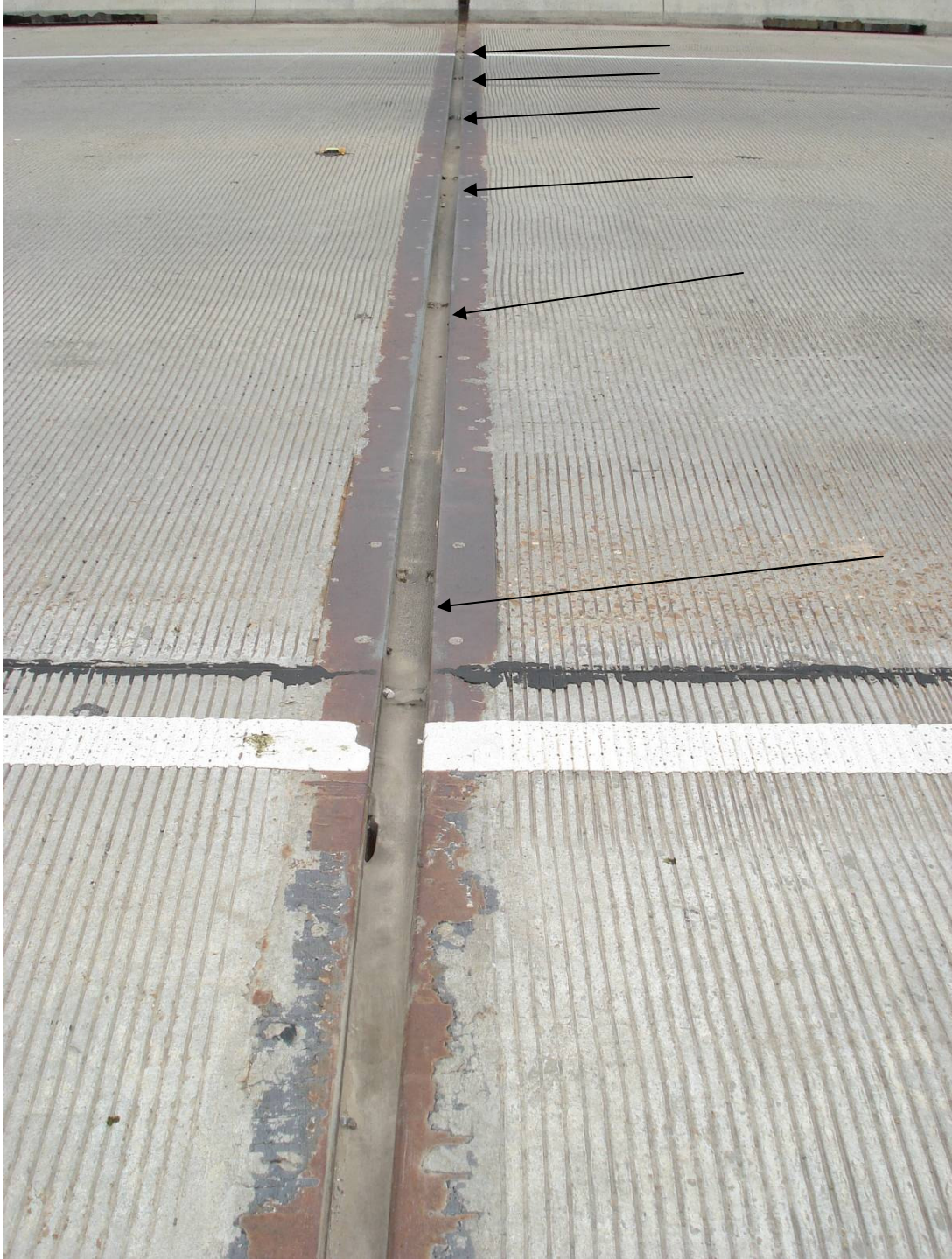
Figure 26: Cache River Interval Tearing/Detaching of Silicone Joint
