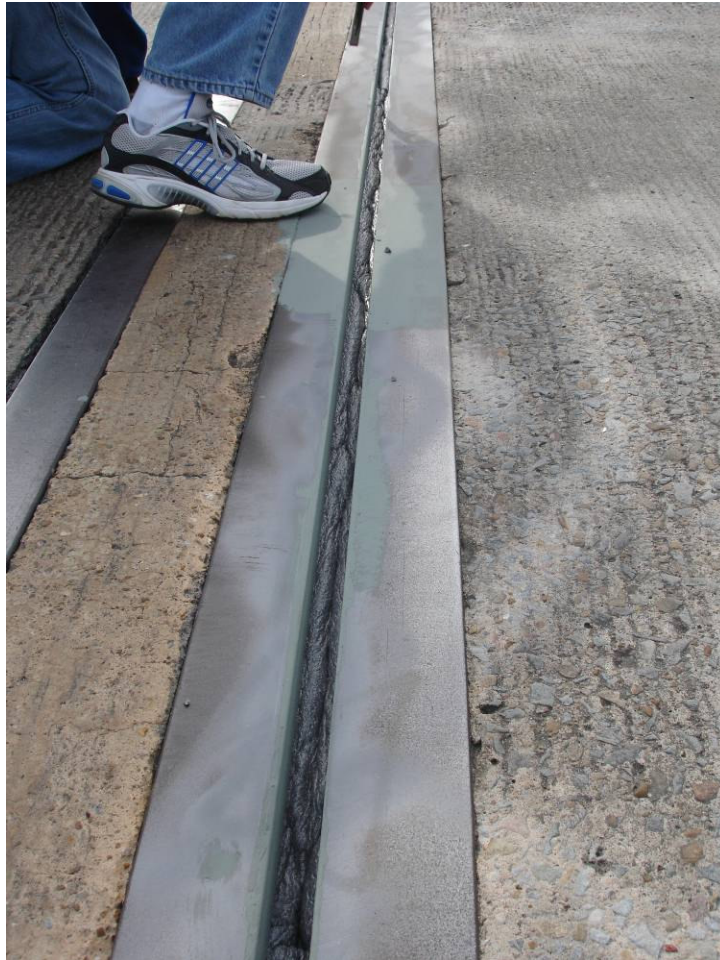
Figure 31: Bald Knob Exit 54 "Wrinkly" Backer Rod in Joint
