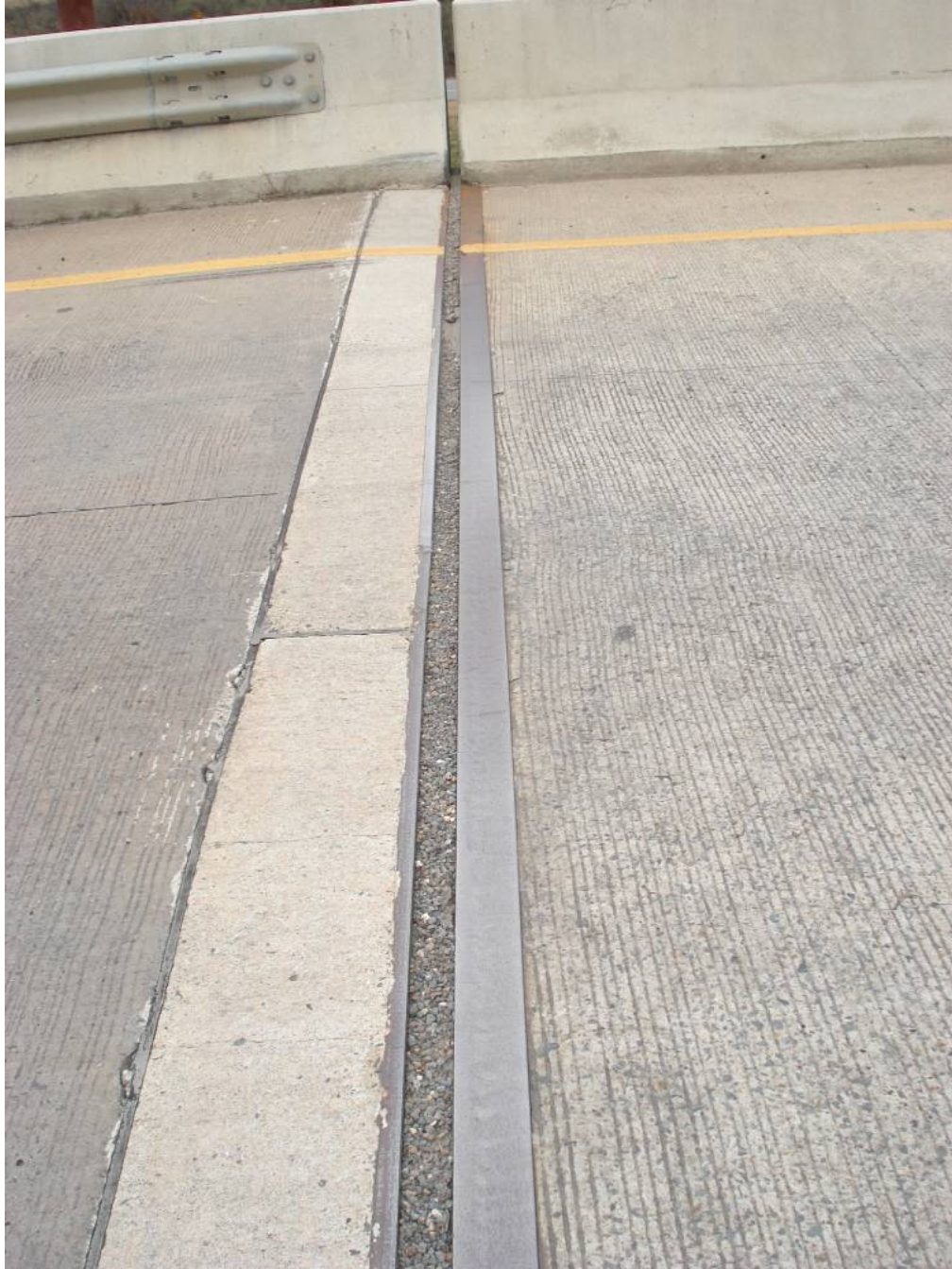
Figure 27: I-440 Interchange Debris Build-up on Joint
