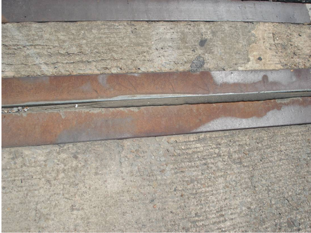
Figure 32: Bald Knob Exit 54 Joint Sealant Pushing Up to Roadway (8-9-07)
