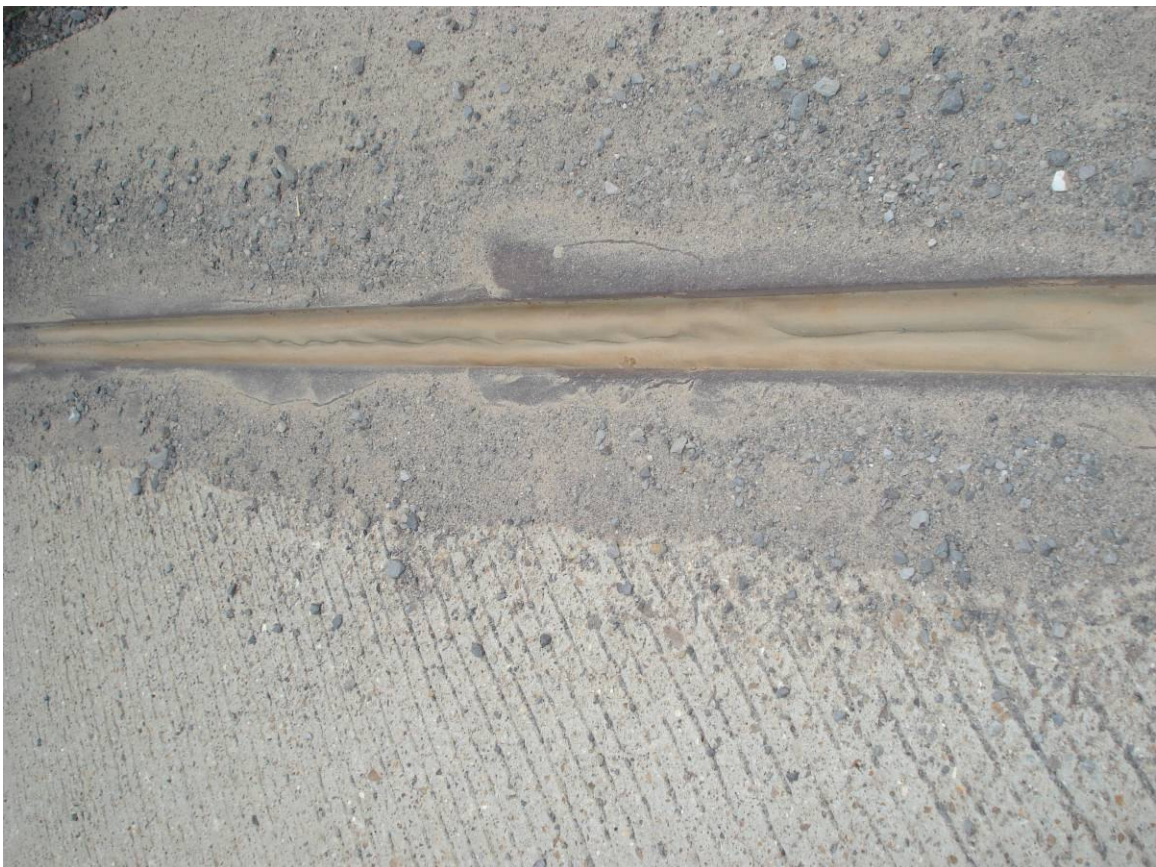
Figure 24: Caddo River County Road "Wrinkly" Joint
