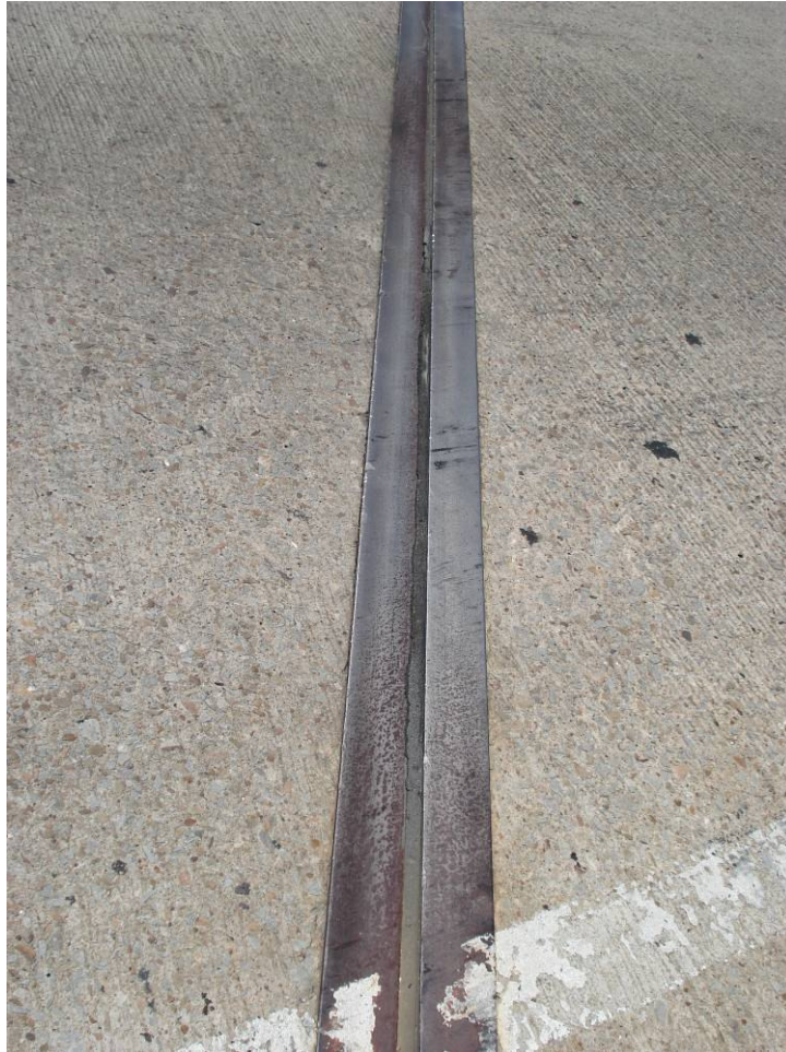
Figure 33: Southbound Creek Bridge Joint Damage (8-9-07)
