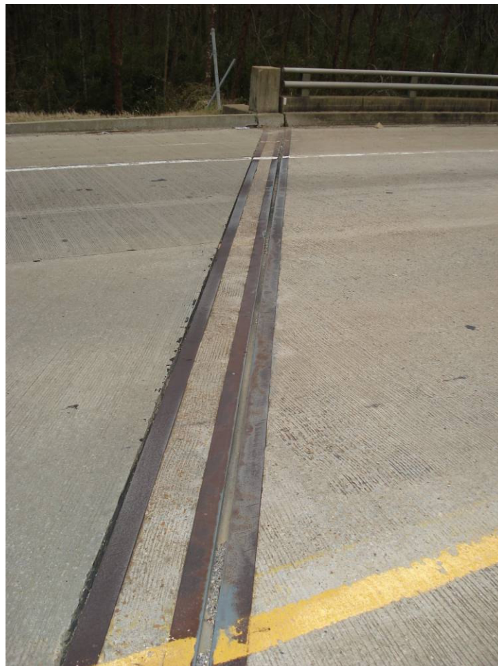
Figure 34: Bald Knob Northbound Creek Joint (1-16-08)
